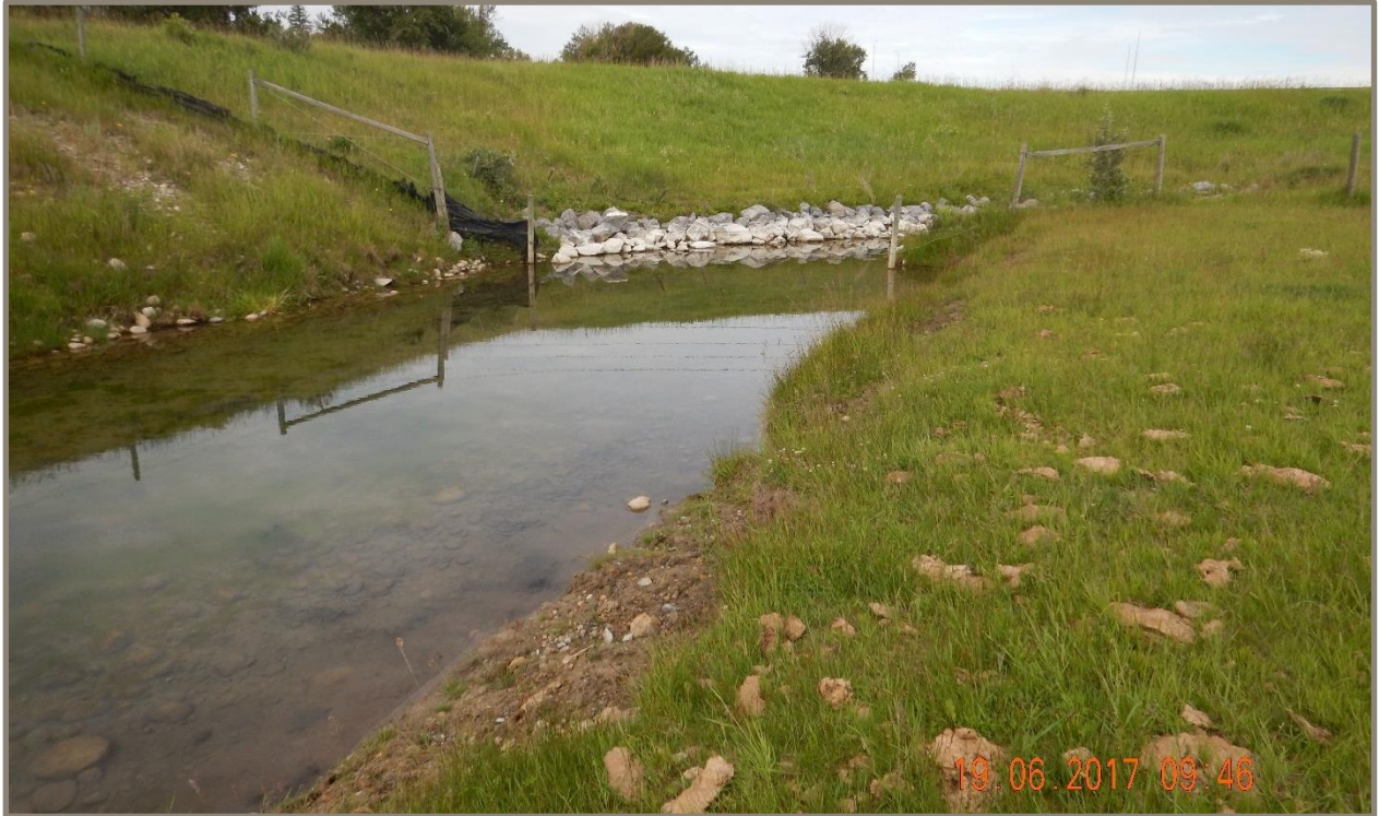
PHOTO 5.16: VIEW WEST OF NORTHWESTERN PORTION OF A02 CHANNEL SHOWING WATER AND RIPRAP
